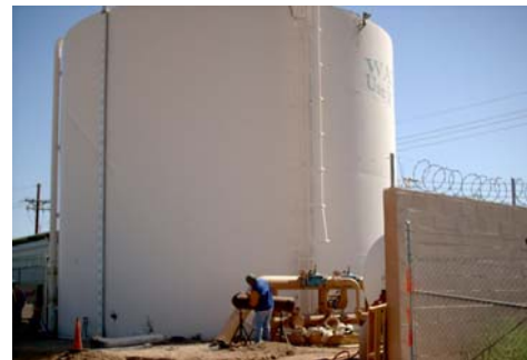
Metro Water's South Shannon Well and Water Tank
