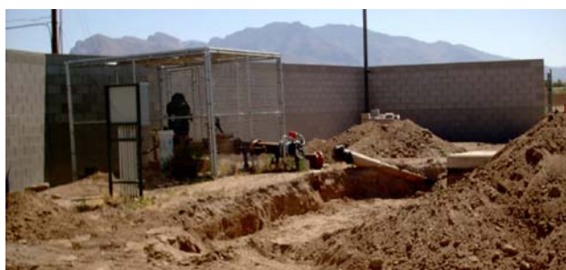
Upgrading the Treatment System at the South Shannon Well
