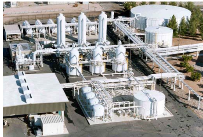
Air Force Plant 44 Groundwater Treatment Plant
