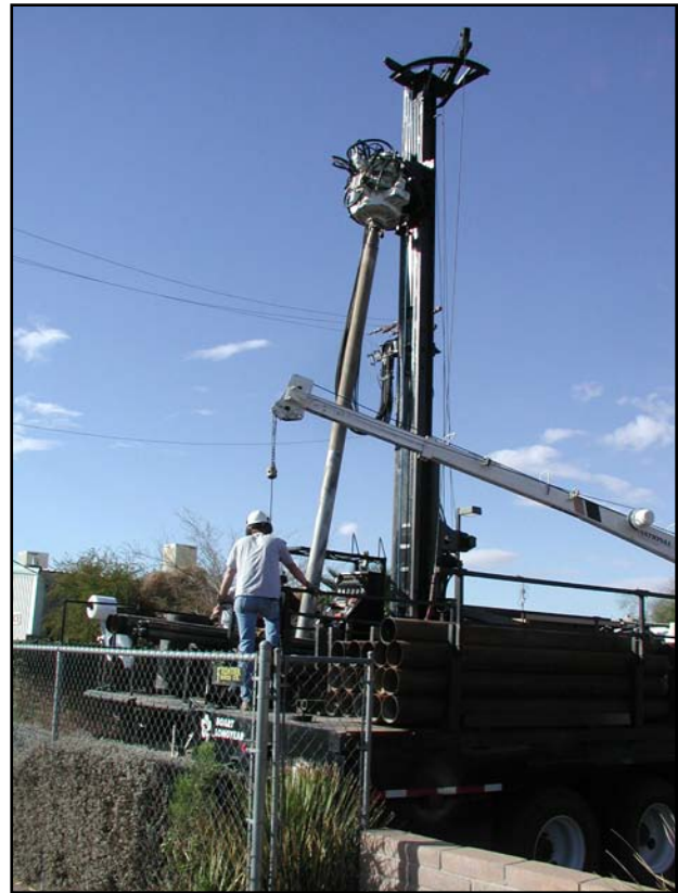
Several monitor wells have been installed to investigate the contamination in and around the Miracle Mile WQARF site.
