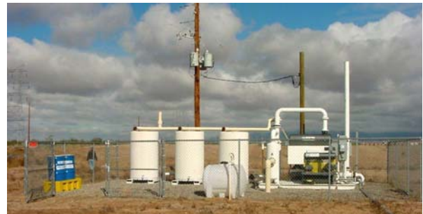
The Soil Vapor Extraction System at the Southwest Disposal Area
