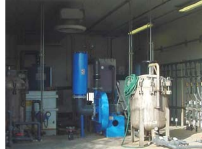
The Pump and Treat System at the Los Reales Landfill
