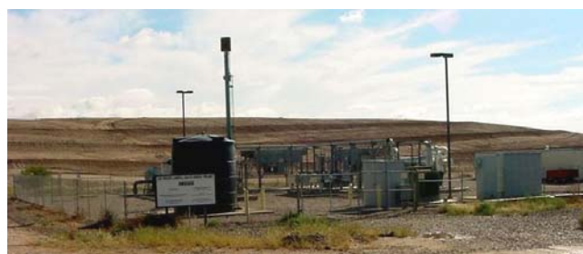
Landfill Gas Piped to Tucson Electric Power
