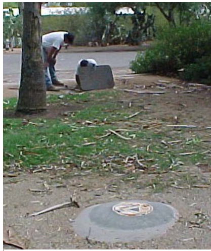
Monitor Well on Residential Street Right-of-Way
