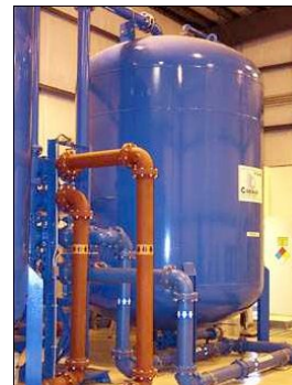
Carbon Chamber at EGTS
